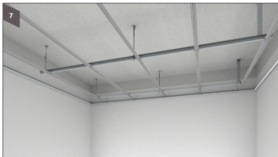
Connect the spring tee to the primary channel at 600 spacing using wire connecting clip WCC
